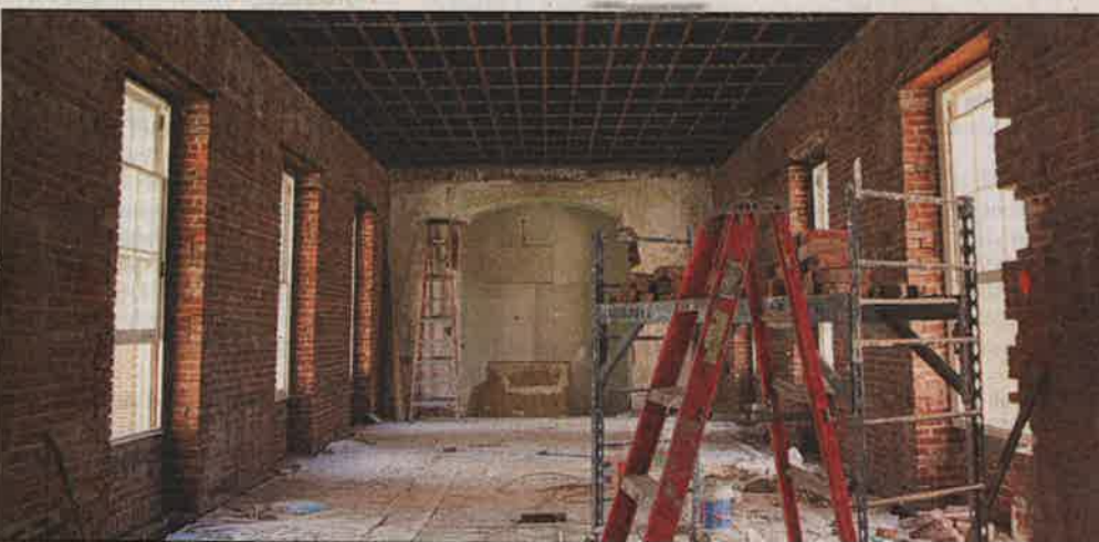
For the retrofitting, many interiors in the 1879-building were stripped to bare brick.
